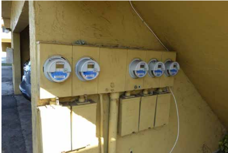
Above: Typical a/c units for each fourplex Below: Typical four units meters and house meter for each fourplex unit
