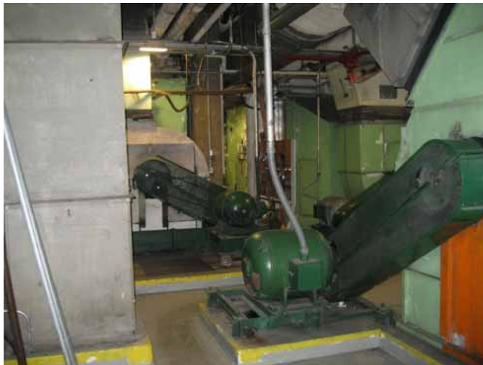
TYPICAL ROOF MECHANICALS
