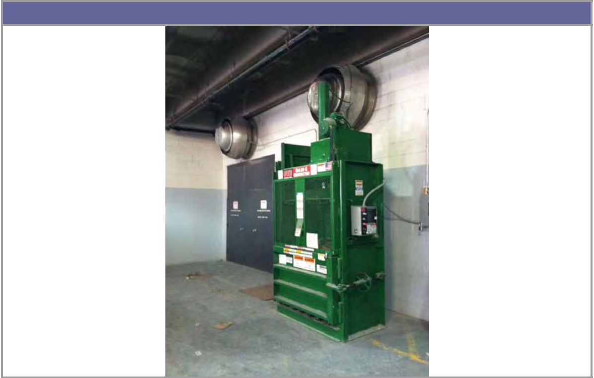
Loading Dock: Box Compactor
